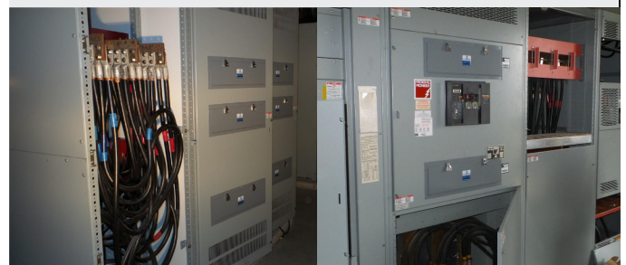
Incoming line connection and main breaker cabinets were also fitted with 24-inch windows
